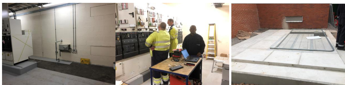
Figure 8: 11kV Switchroom at UoW Primary before installing new panels (left), after installation of new panels (middle) and completed FCLi foundation (right)
