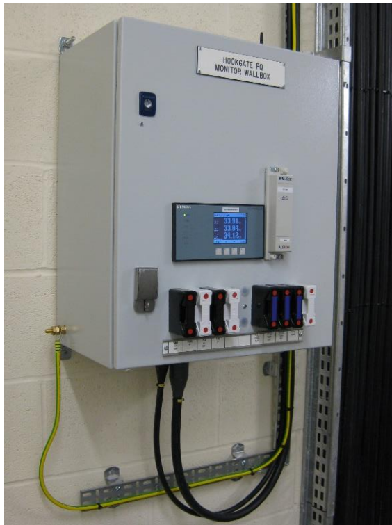
(a) PQ panel with PQ monitor
