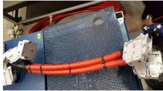
Figure 5: 11kV 3-core Trefoil XLPE cable
