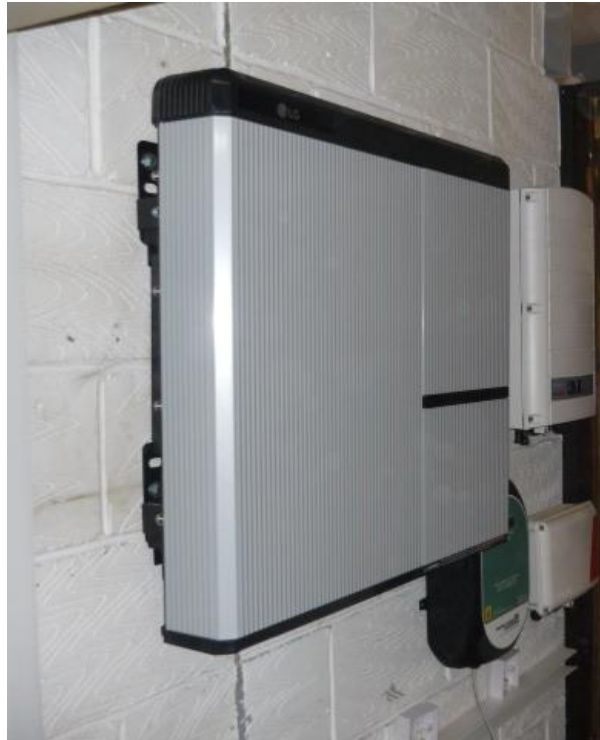
Figure 2-3: Example Installation of Project Equipment: A Controllable EV Charge Point and Domestic Load Controller
