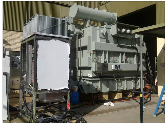
Figure 1: PSCFCL during short-circuit testing in Sydney, Australia
