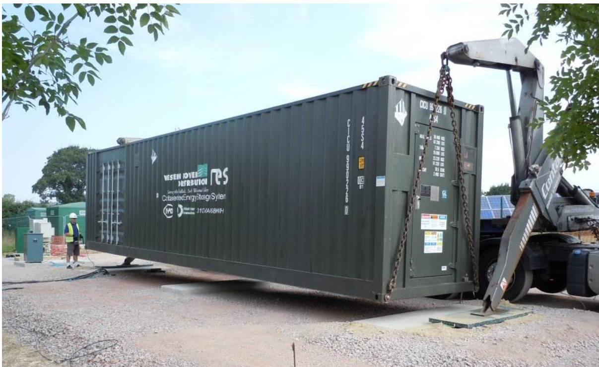
Image 3 - Battery installation / delivery
