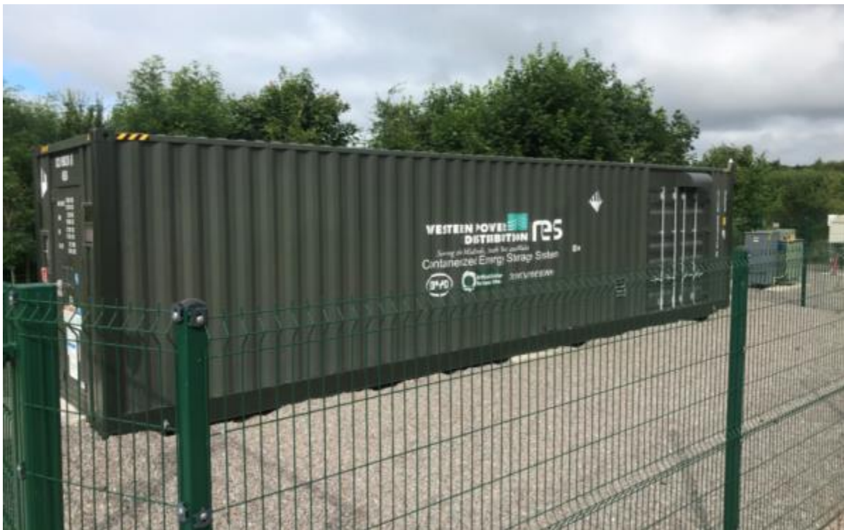
Image 5 - Fully operational installation with security fencing
