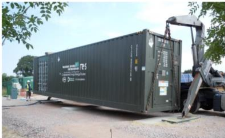
Image 3 - Battery installation / delivery
