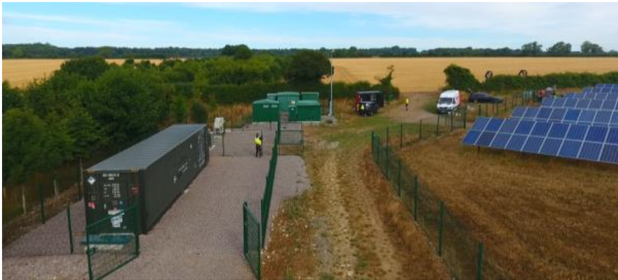
Image 8 - Site access to battery
