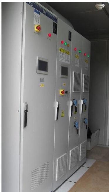
Left – Circuit breakers and emergency stop.
