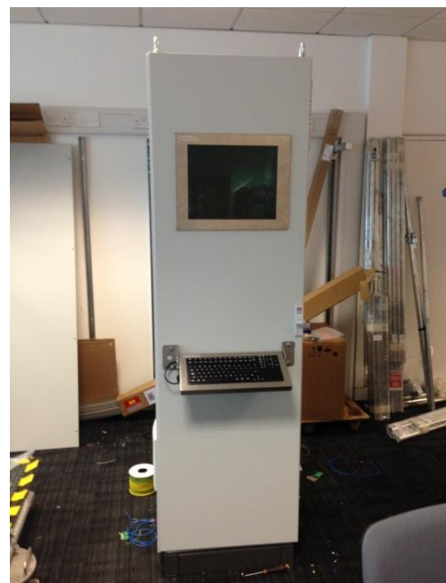
Right – Resolve control panel.
