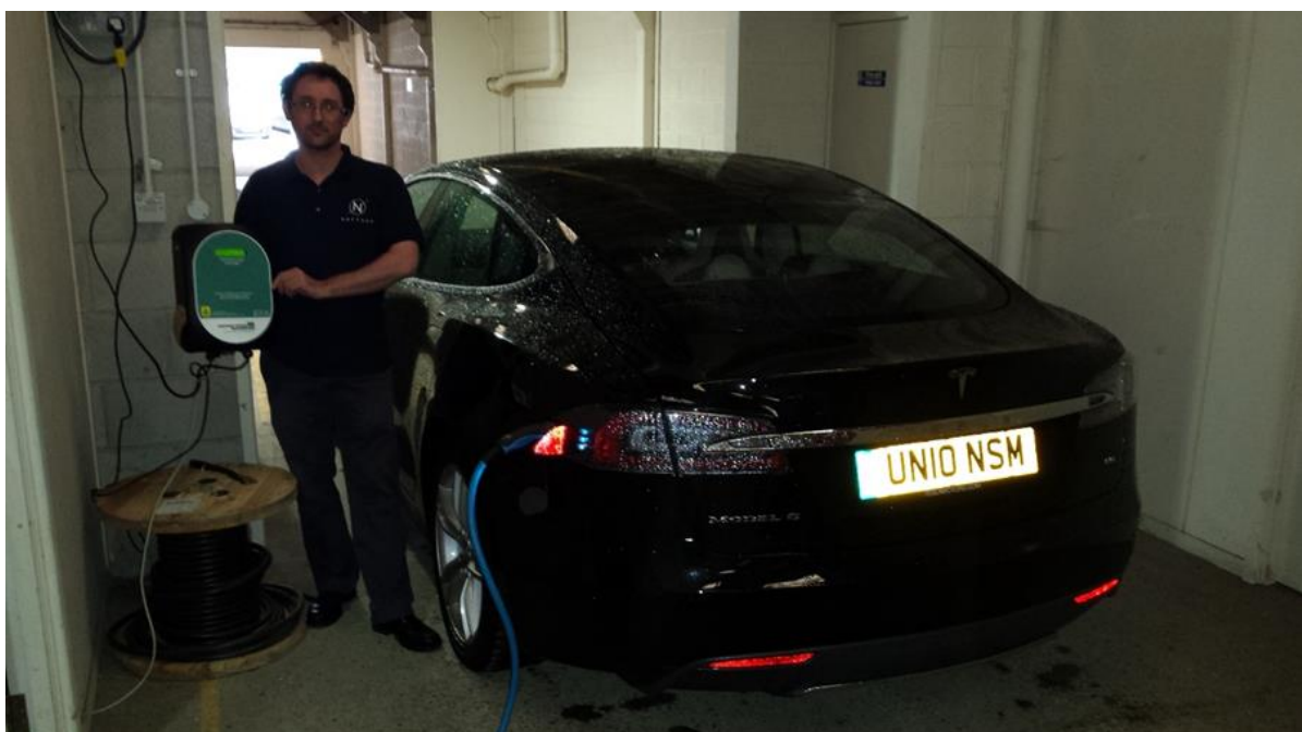
DLC Box / EV Charge Point Testing with a Tesla Model S
