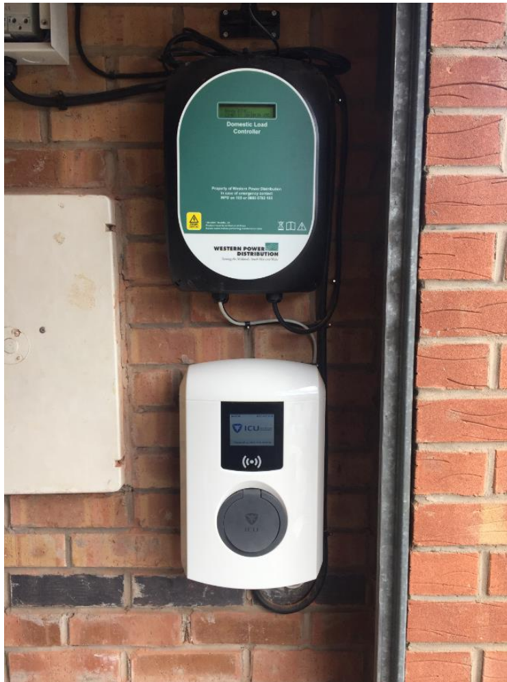
Typical EV charger customer installation
