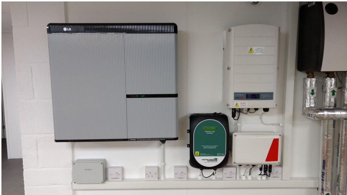
Battery/Inverter system installed as a test rig at Stratford Energy
