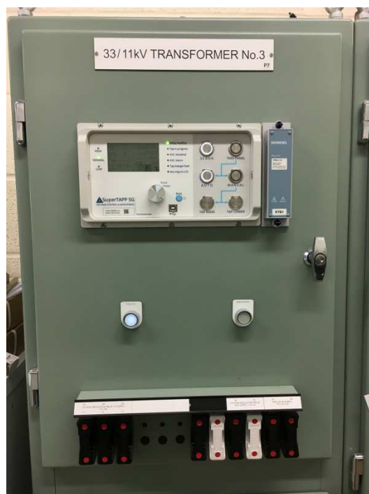
Figure 2-7: Picture of T3 AVC Panel with SuperTAPP SG Installed
