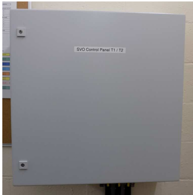
Figure 2-11: SVO MicroTAPP Control Panel at Lydeard St Lawrence
