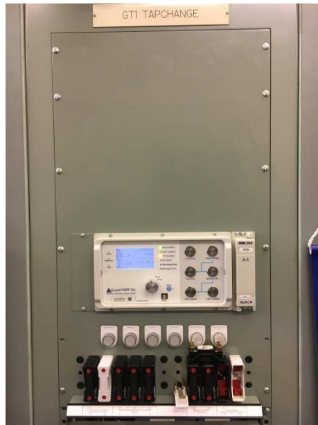
Figure 2-10: Paignton GT1 SuperTAPP SG during commissioning
