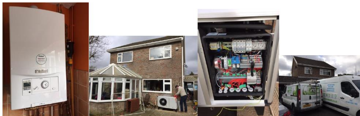
Figure 4: MasterTherm heat pump
