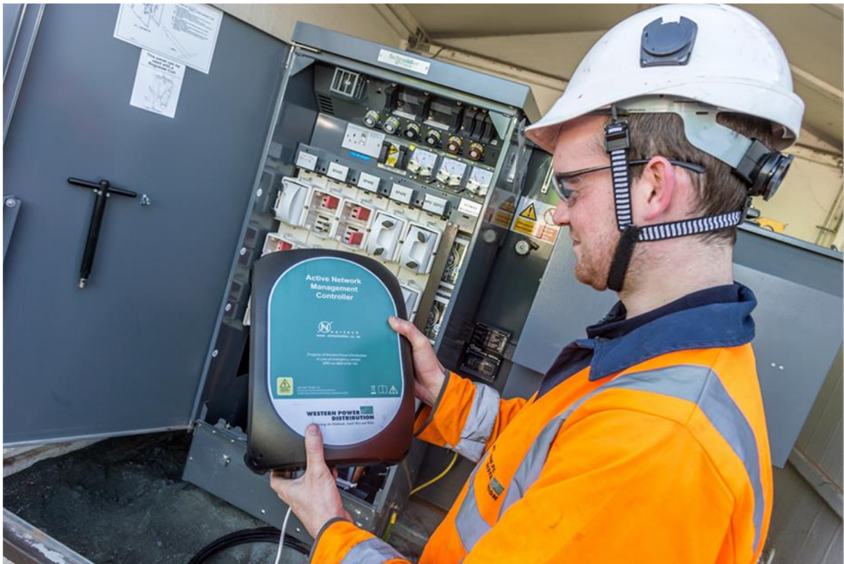
Above: WPD fitter inspects the Active Network Management Controller installed at WPDs Hereford Depot
