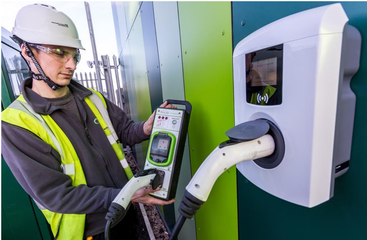
Above: WPD fitter tests the EV charging device installed at WPDs Hereford Depot
