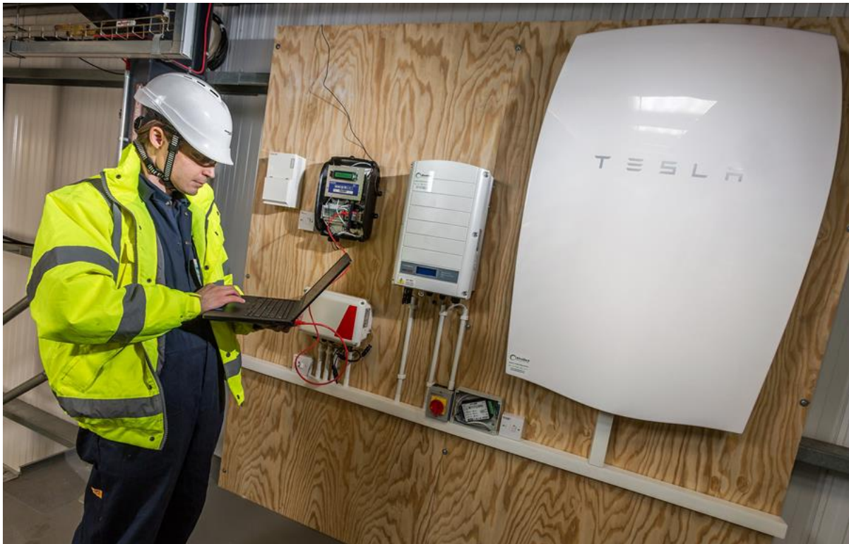
Above: WPD fitter configures the Battery Storage system installed at WPDs Hereford Depot.
