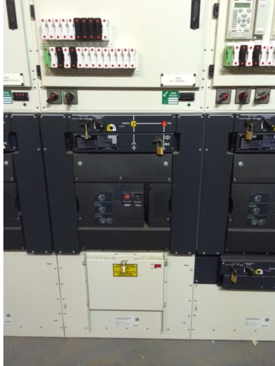
Figure 6-1 - 11kV S/Gear for FLM and FCL
