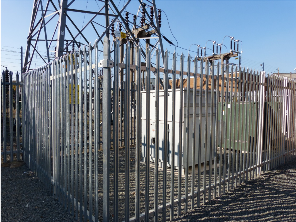
Figure 6-2 - FLM 11kV Compound
