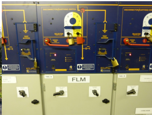
Figure 6-2 - FLM 11kV Circuit Breaker
