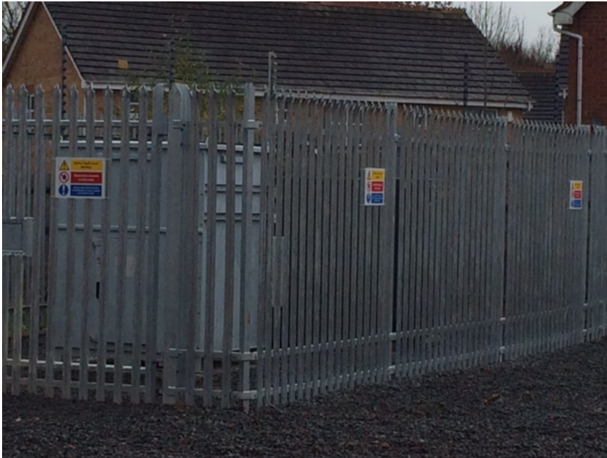
Figure 6-1 - FLM 11kV Compound
