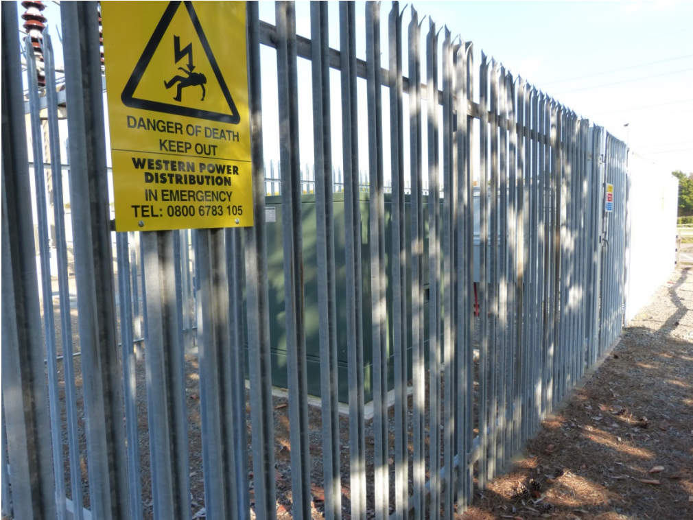
Figure 6-3 - FLM 11kV Compound
