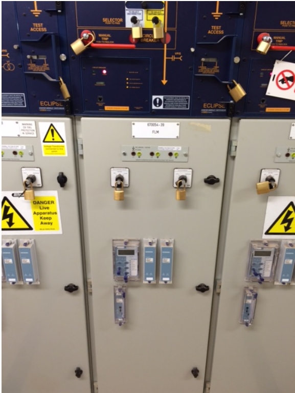
Figure 6-3 - FLM 11kV Circuit Breaker
