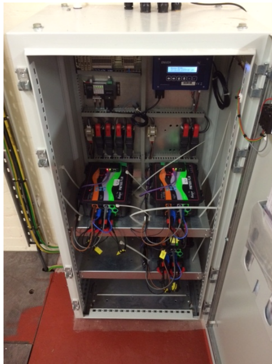
Figure 6-3 - FLM Control Cubicle (Internal)
