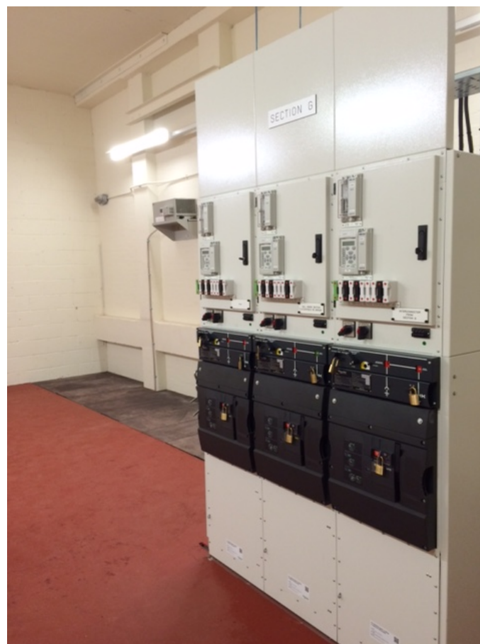
Figure 6-1 - FLM 11kV Circuit Breakers
