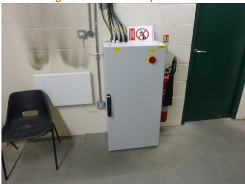
Figure 6-3 - FLM Control Cubicle
