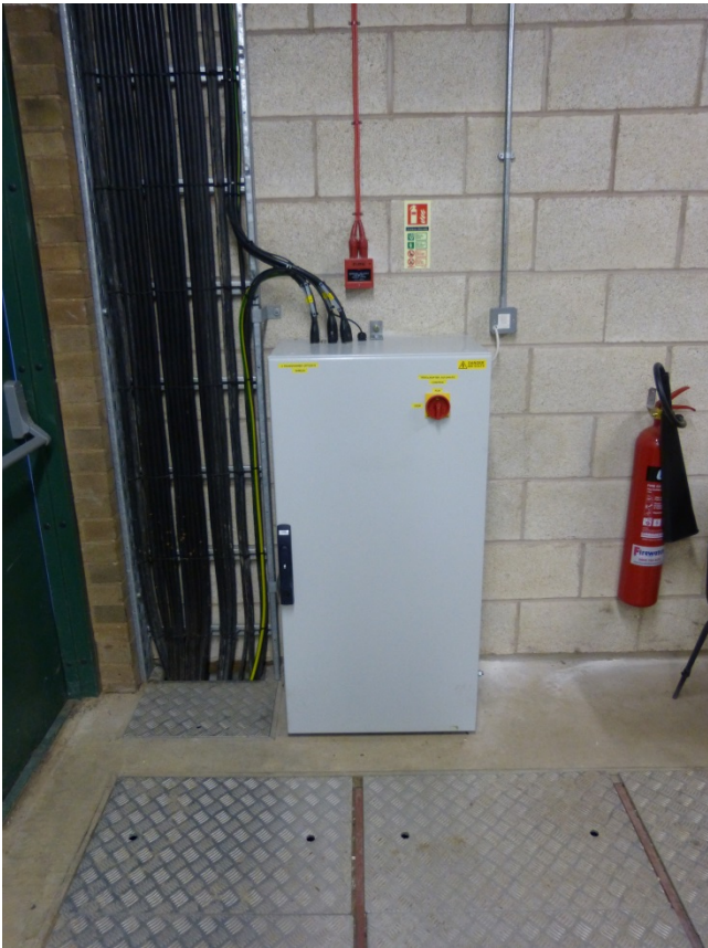
Figure 6-1 - FLM Control Cubicle
