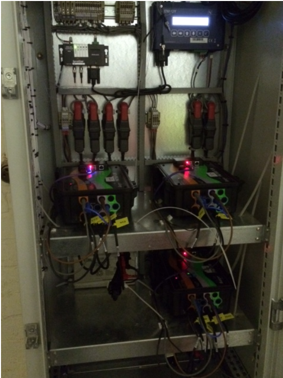
Figure 6-4 - FLM Control Cubicle (Internal)
