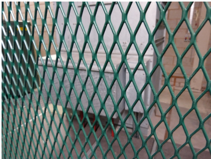
Figure 6-2 - FLM 11kV Compound
