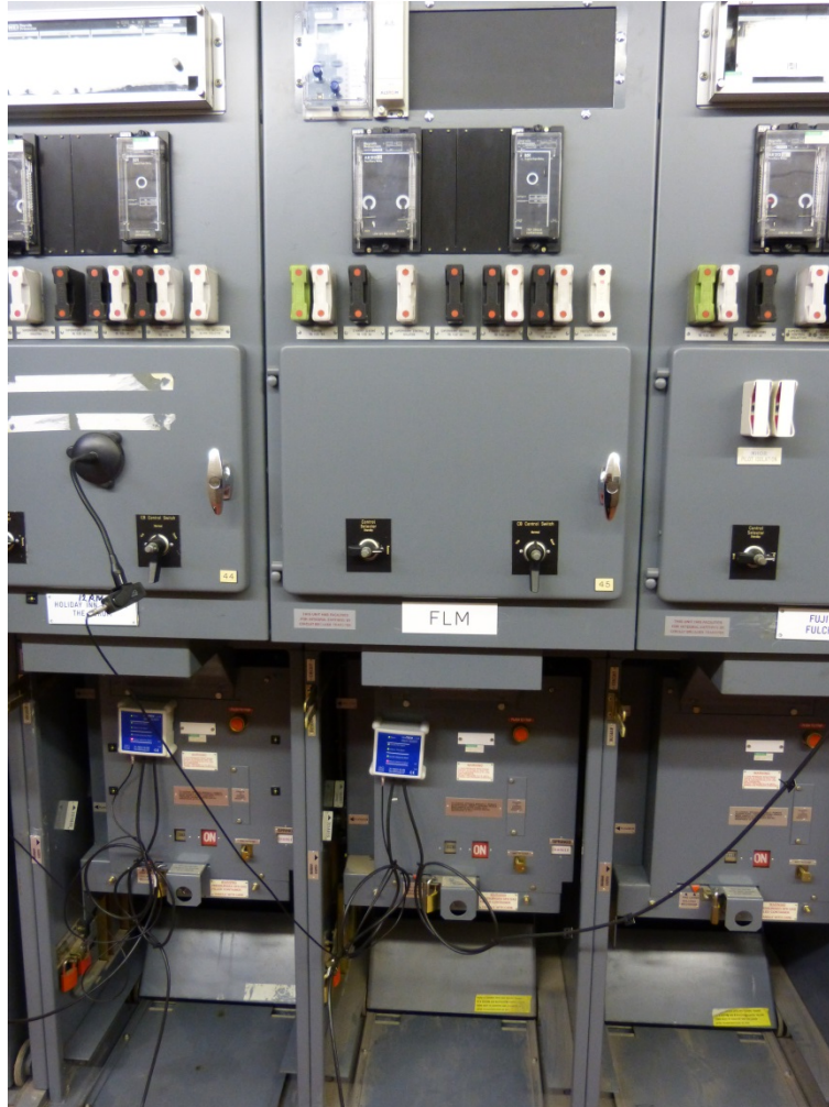
Figure 6-1 - FLM 11kV Circuit Breaker
