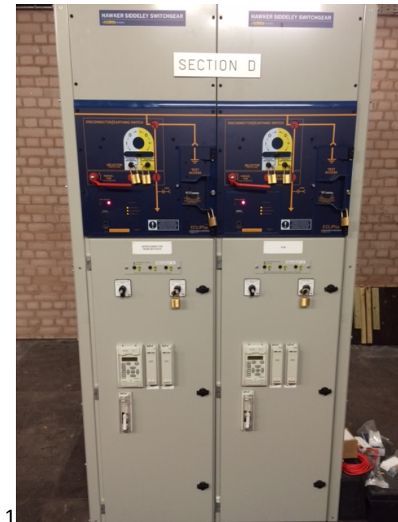
Figure 6-2 - FLM 11kV Circuit Breakers
