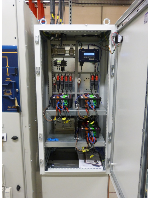
Figure 6-1 - FLM Control Cubicle Internal
