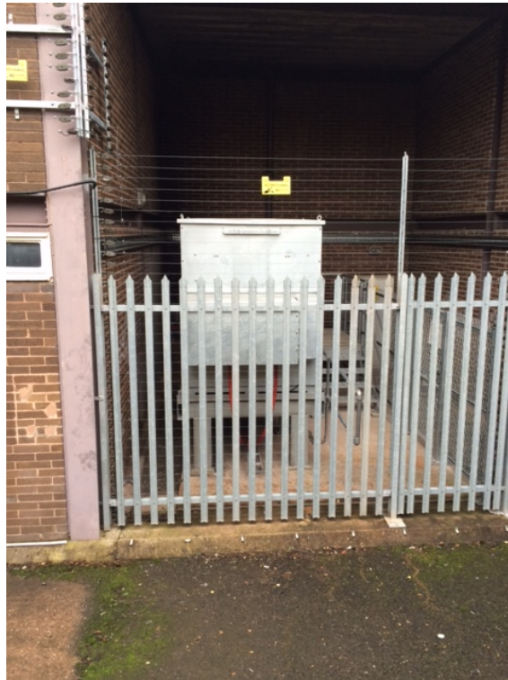
Figure 6-3 - FLM 11kV Compound
