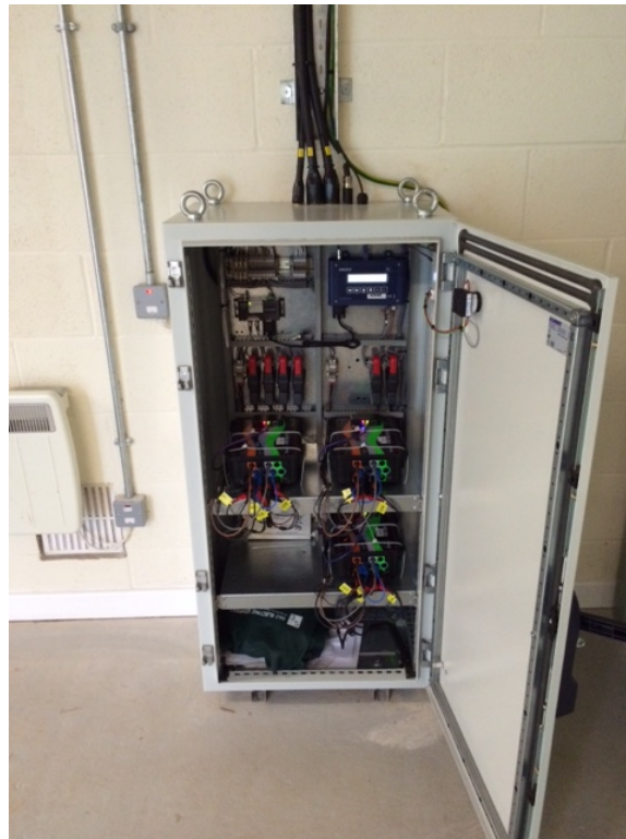
Figure 6-2 - FLM Control Cubicle (Internal)
