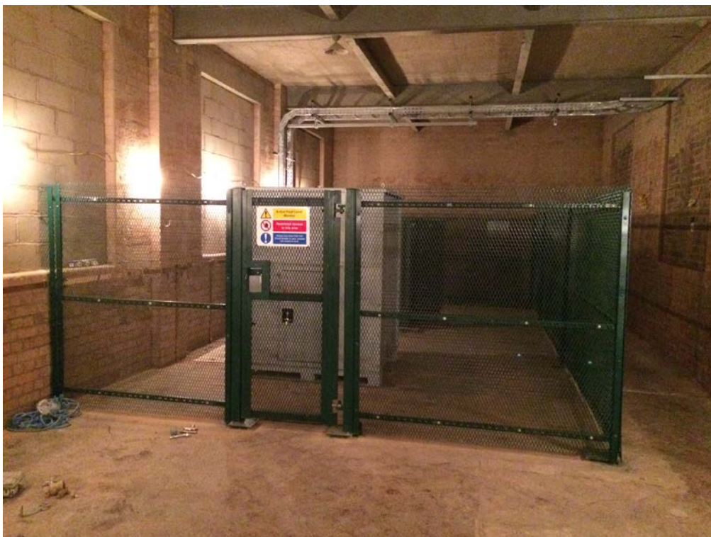
Figure 6-2 - FLM 11kV Compound
