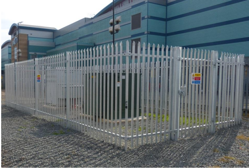
Figure 2-1 - PMIR and Resistor installed at Nechells West Substation
