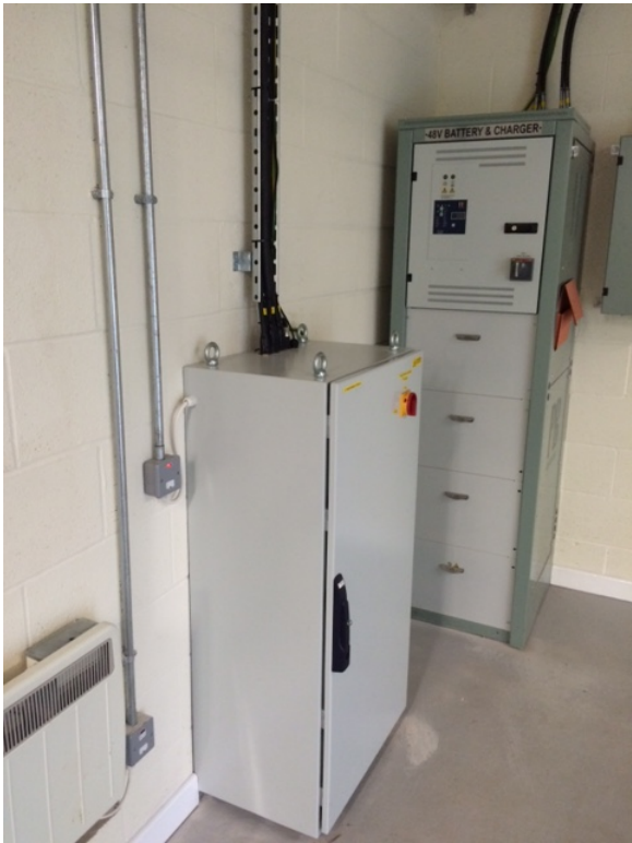
Figure 6-3 - FLM Control Cubicle
