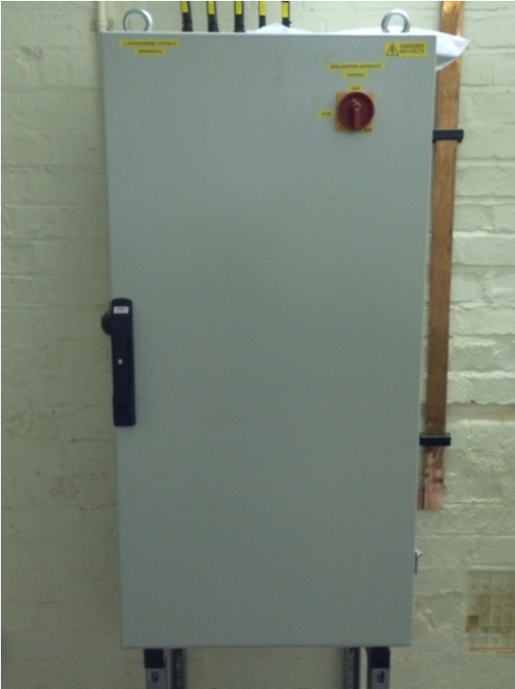
Figure 6-3 - FLM Control Cubicle
