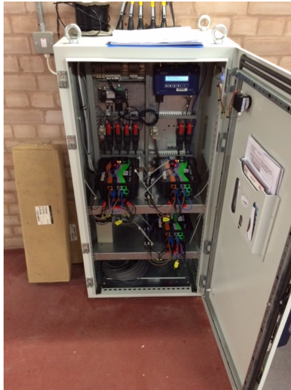
Figure 6-1 - FLM Control Cubicle (Internal)
