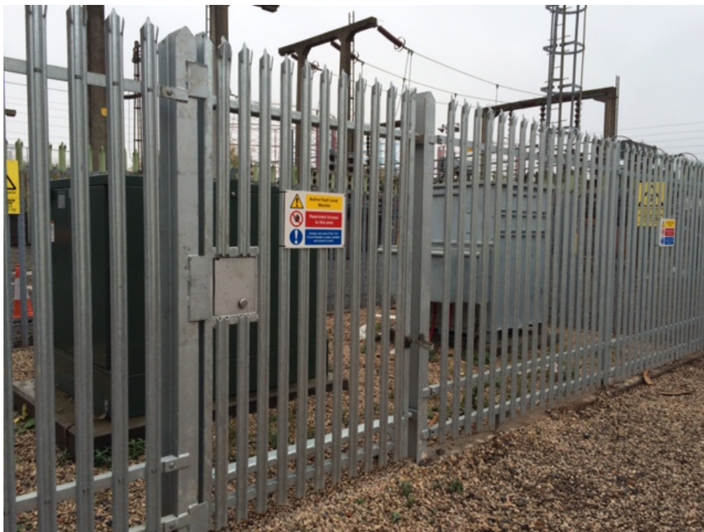
Figure 6-1 - FLM 11kV Compound
