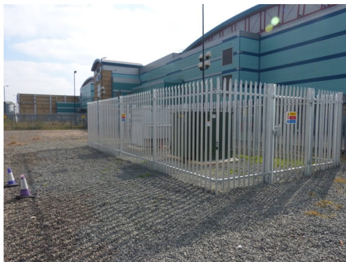
Figure 6-2 - FLM 11kV Compound
