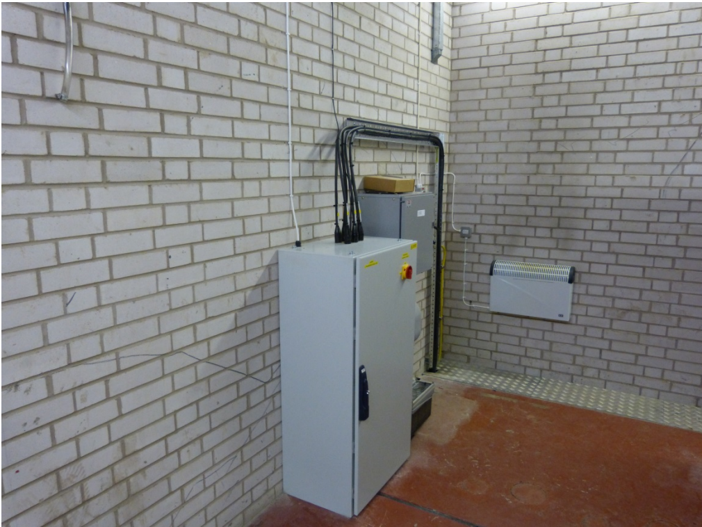
Figure 6-2 - FLM Control Cubicle
