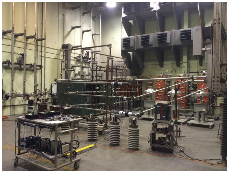
Figure 4-3 - Test Lab during FL Tests
