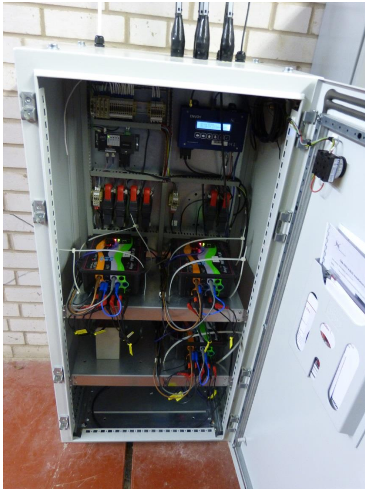
Figure 2-2 - 3 off PM7000s and Envoy installed in FLM Control Cubicle
