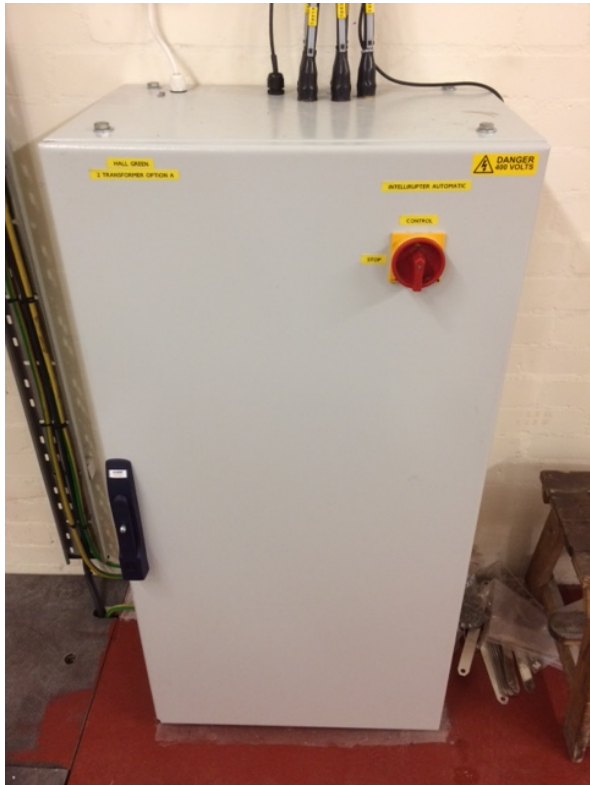
Figure 6-2 - FLM Control Cubicle
