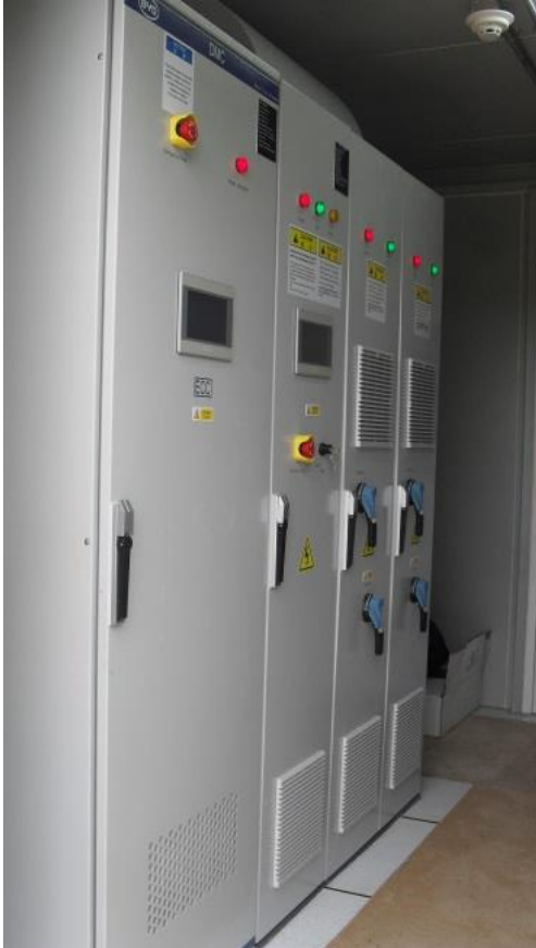
Circuit breakers and emergency stop
