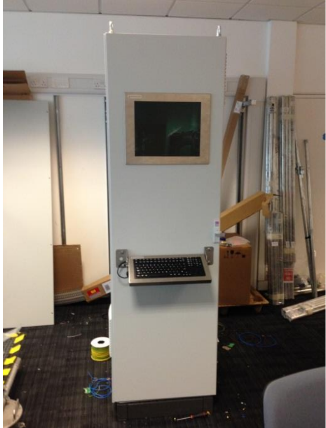
Resolve control panel
