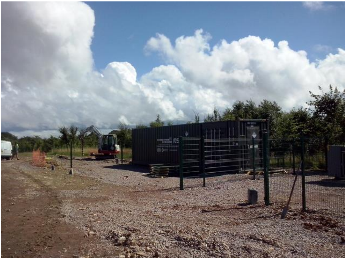
Battery on the plinth before and after fencing
