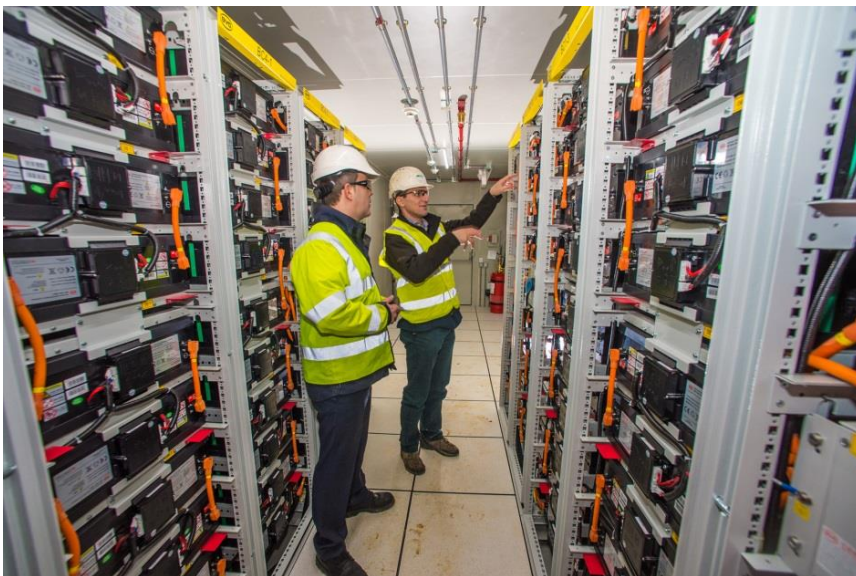
Battery strings and fire suppression system
