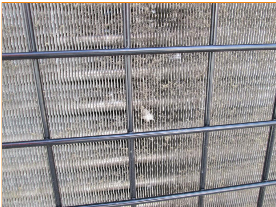
Figure 4-7: Photograph of the debris obstructing the air flow to the cooler condenser
