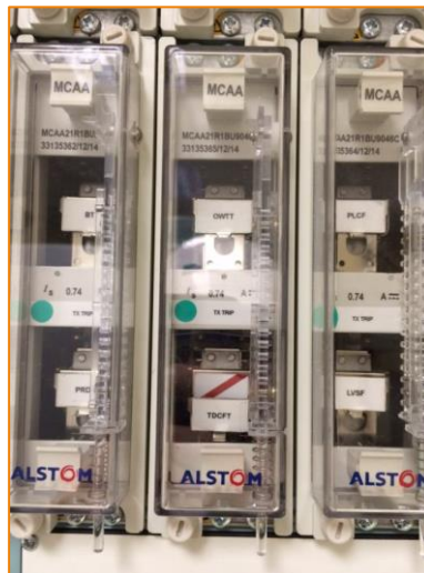
Figure 4-2: TDCFT trip alarm relay on PSCFCL protection panel
