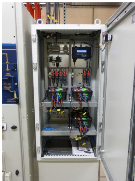
Figure 3-1 - FLM Control Cubicle
