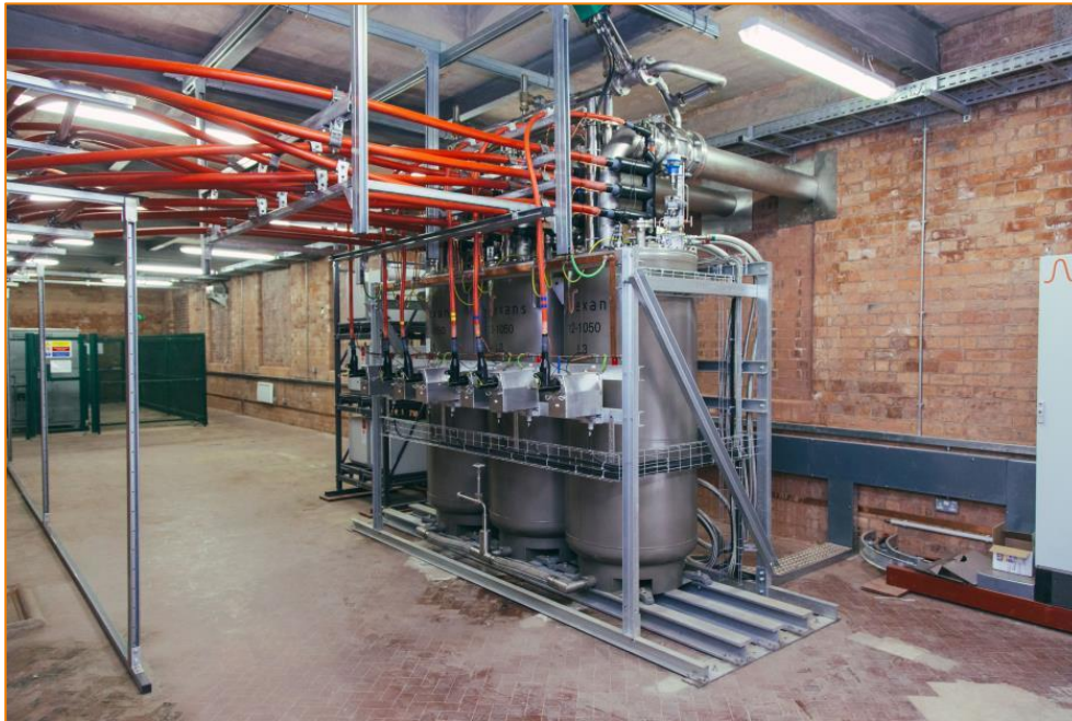
Figure 8-2: Photograph of the complete FCL installation at Bournville
