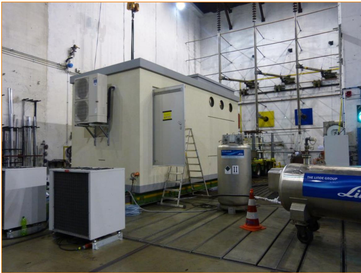
Figure 6-6: Chester Street FCL during short circuit testing at the KEMA laboratory
