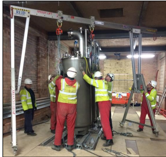
Figure 7-11 – Placement of L2 cryostat vessel in its final position on the first floor
