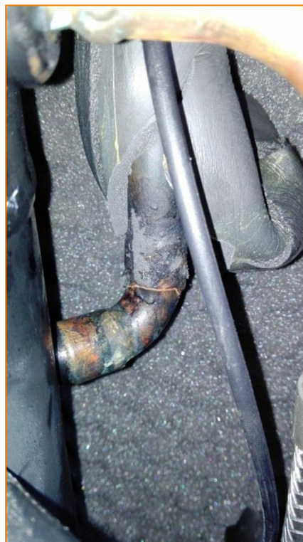
Figure 7-6: Damage to copper pipework in recooling
