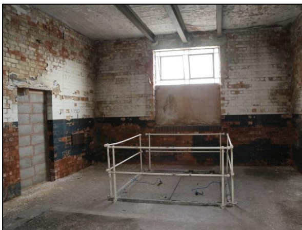
Figure 7-9 – Area above first floor lifting hatch showing lifting beam (top) and sealed emergency exit (left)
