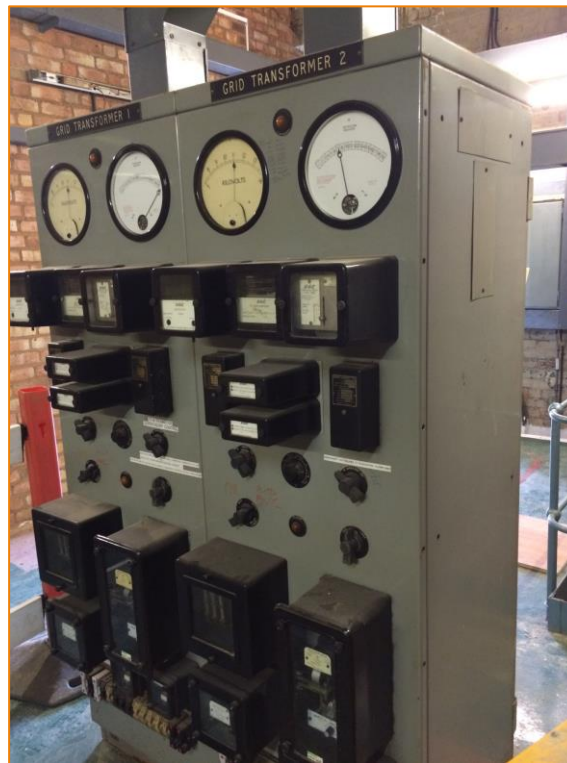
Figure 5-24: Existing AVC relay panels at Bartley Green
