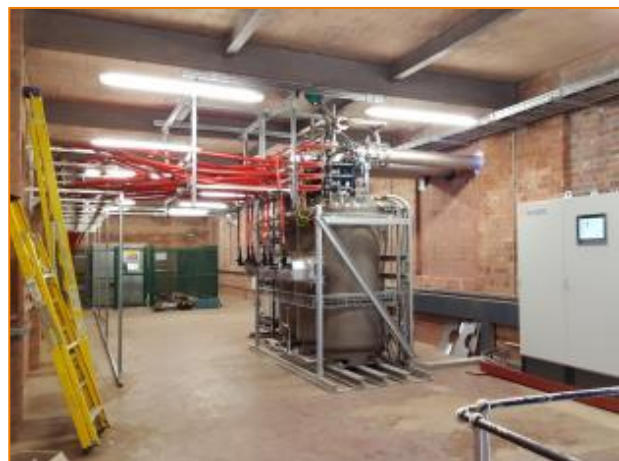
Figure 5-15: View from inside the first floor switchroom after FCL installation
