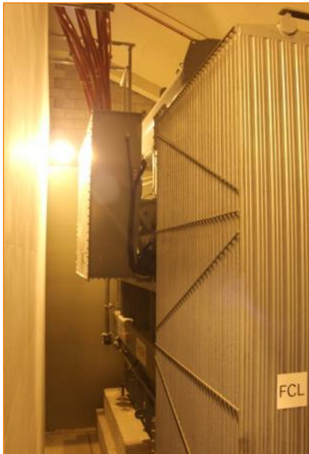
Figure 5-5: Installed FCL with Magnetic Shield covered
