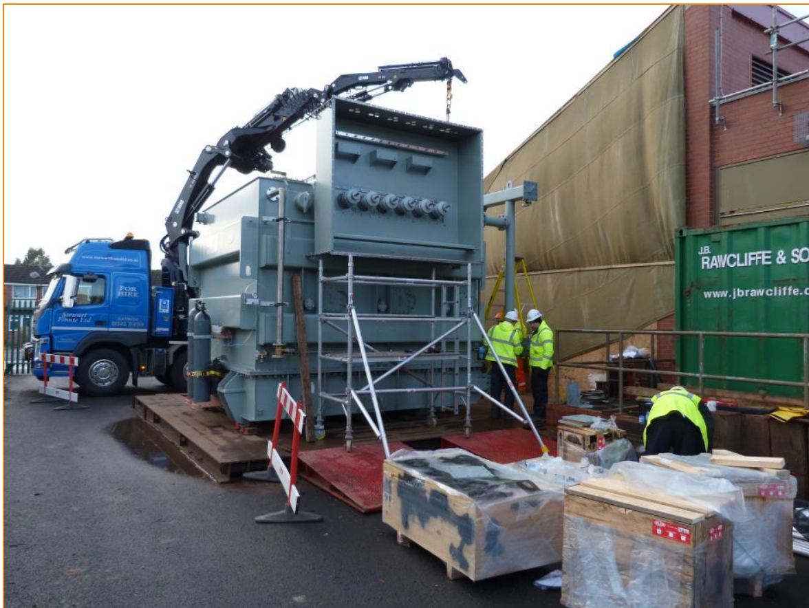
Figure 7-2: Castle Bromwich FCL being prepared for skidding into the spare transformer bay
