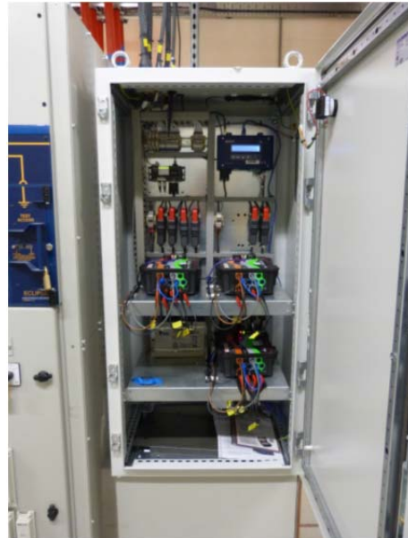
Figure 2-10 - FLM Control Cubicle
