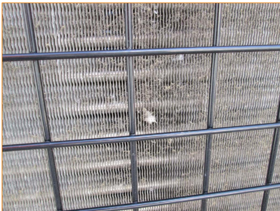
Figure 2-17: Photograph of the debris obstructing the air flow to the re-cooler condenser
