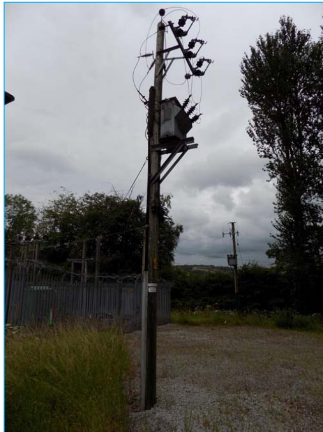
Figure 2-21: Photograph of the existing pole mounted 11/0.415kV transformers supplying Exebridge auxiliary loads
