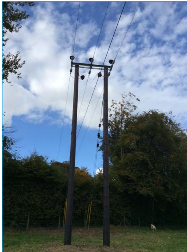
Figure 2-20: Photograph of the new OHL terminal pole on the OHL feeder to Taunton
