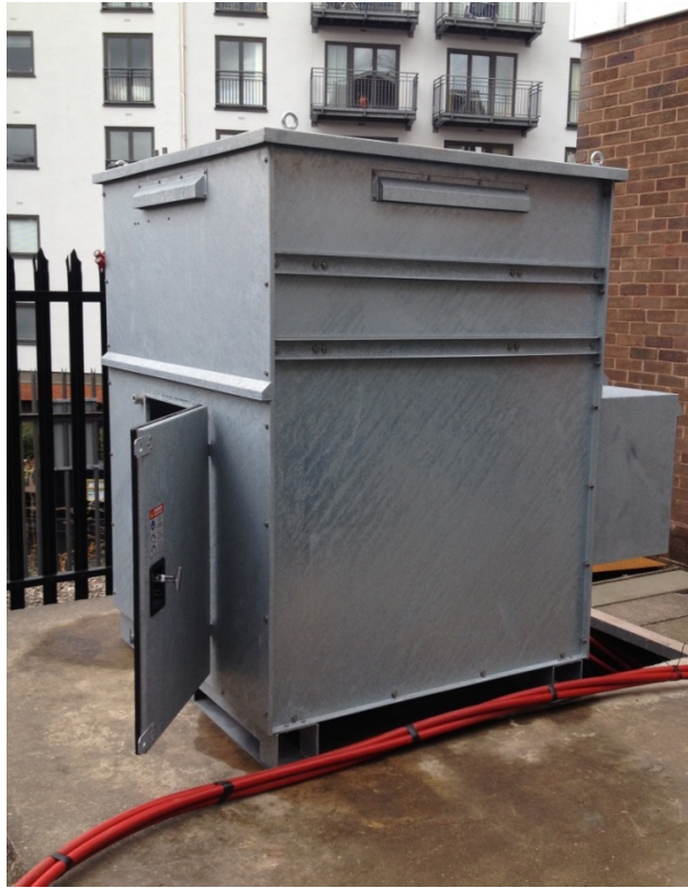
Figure 4-9: Resistor on site
