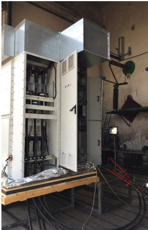
Figure 2-5 FCLi with HV connections in the KEMA test bay
