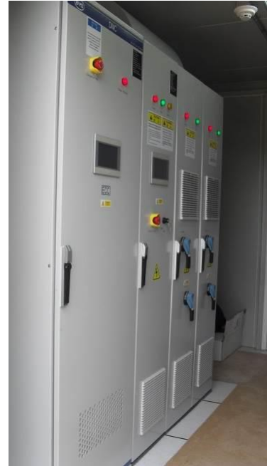
Figure 9: Circuit Breakers and Emergency Stop
