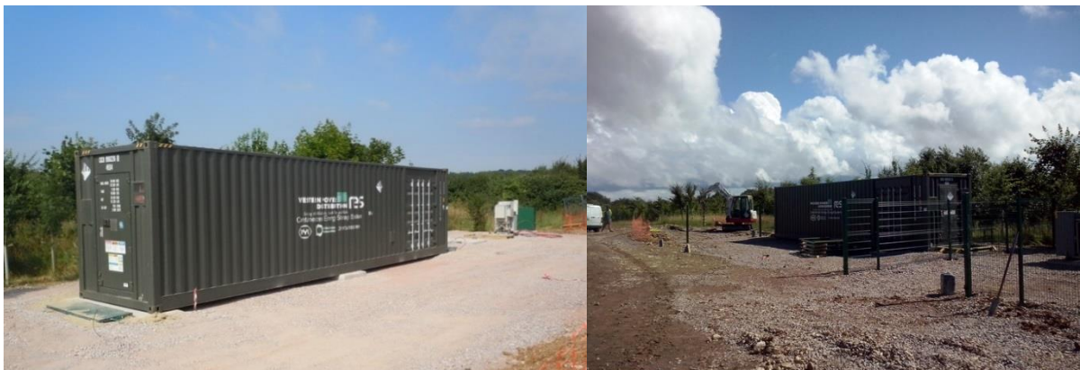
Figure 6: Battery on plinth before and after fencing
