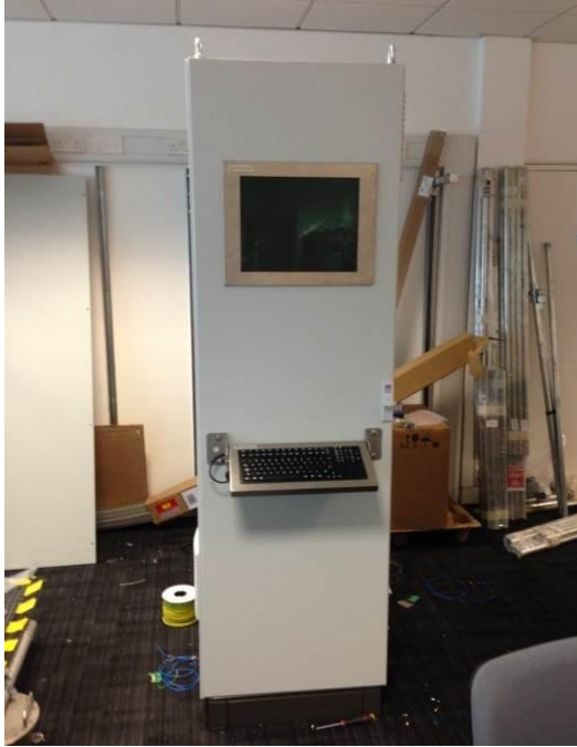
Figure 8: Local Control Panel
