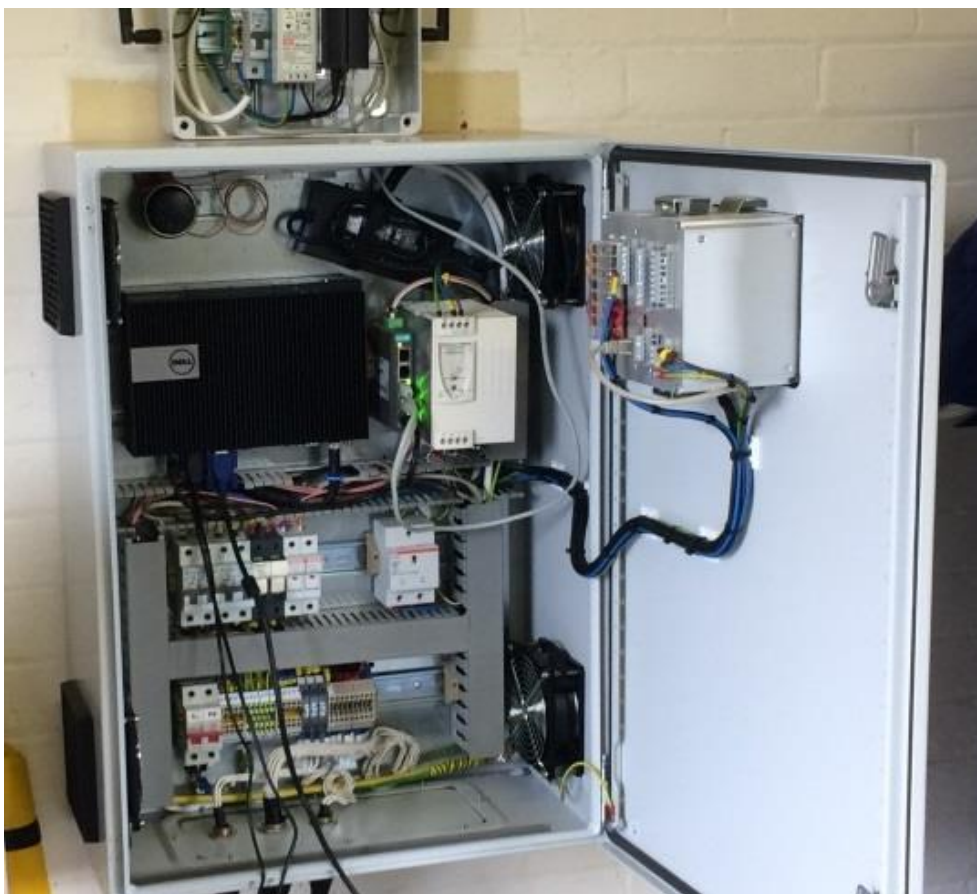
Figure 12: Power quality monitoring and communications equipment installed at Millfield Primary
