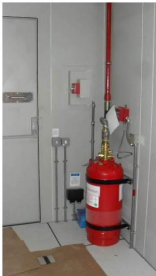
Figure 11: Fire Suppression Equipment
