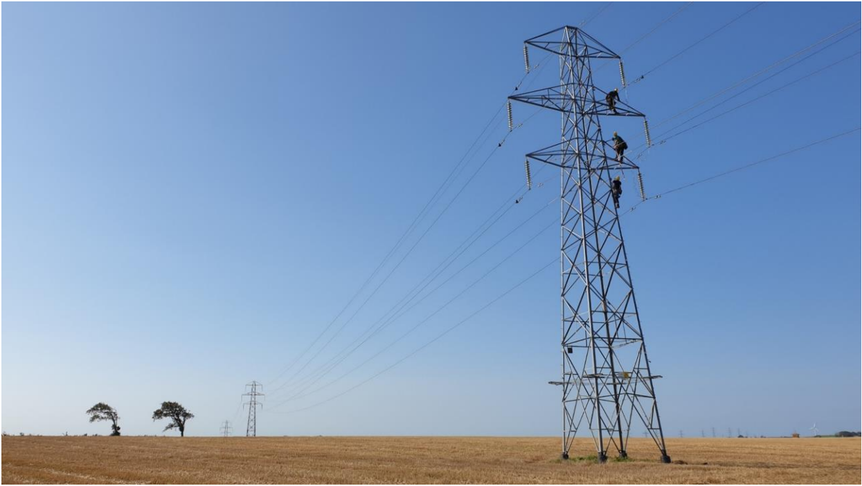
Figure 2-1 – Installations of a set of HV SN2.0 on 132kV K-line tower near to Galsworthy substation
