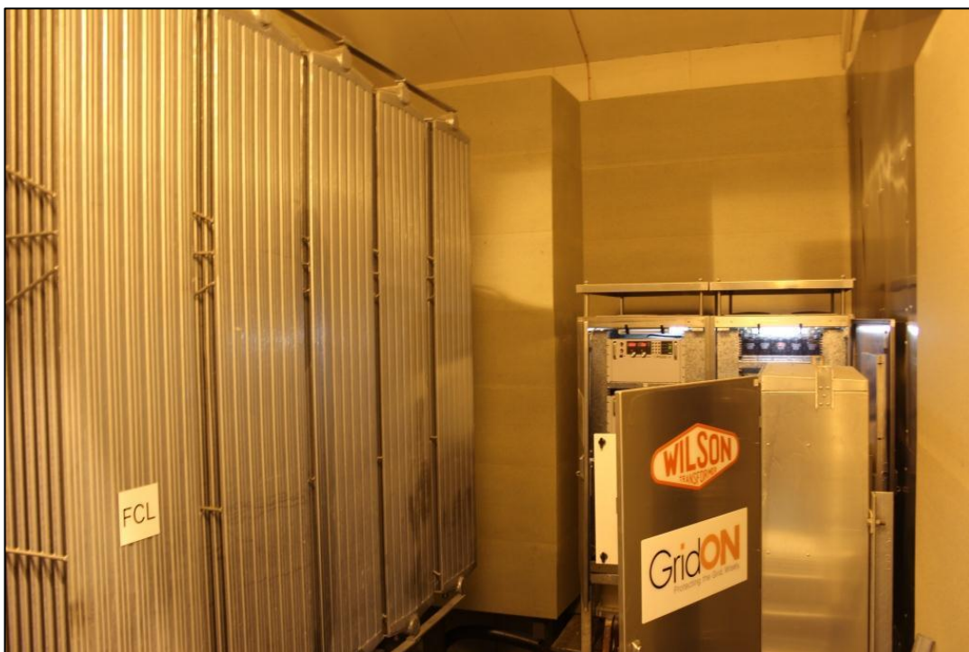
Figure 2-13: Covered magnetic shield around control cabinets
