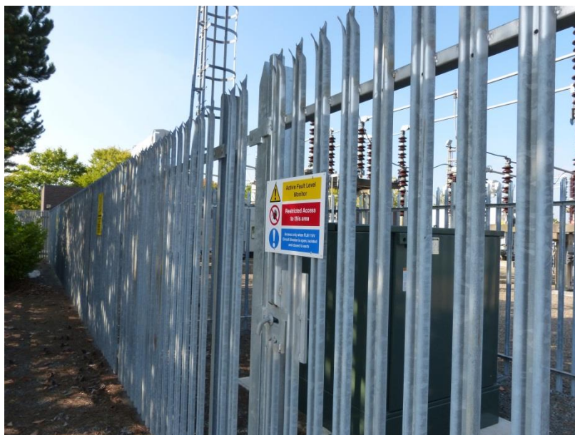
Figure 2-4 - Front view of 11kV FLM
