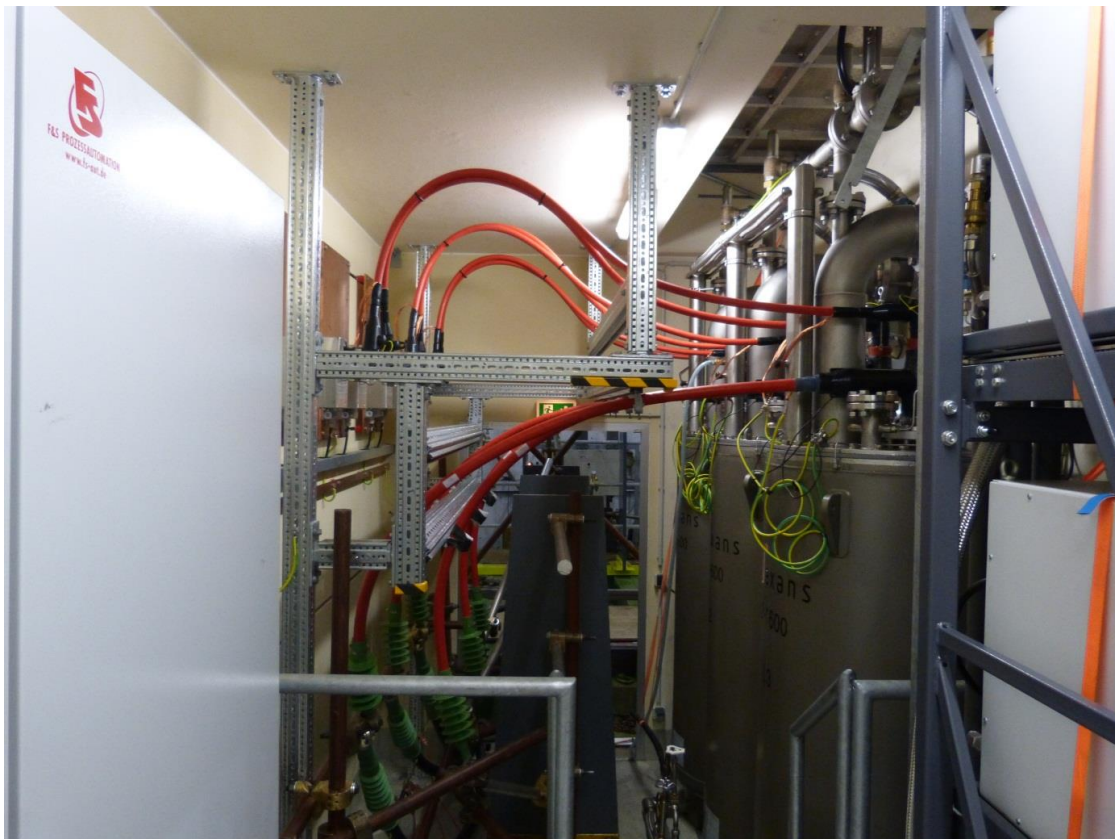
Figure 2-20 - Connections to Chester Street FCL in the KEMA high current laboratory
