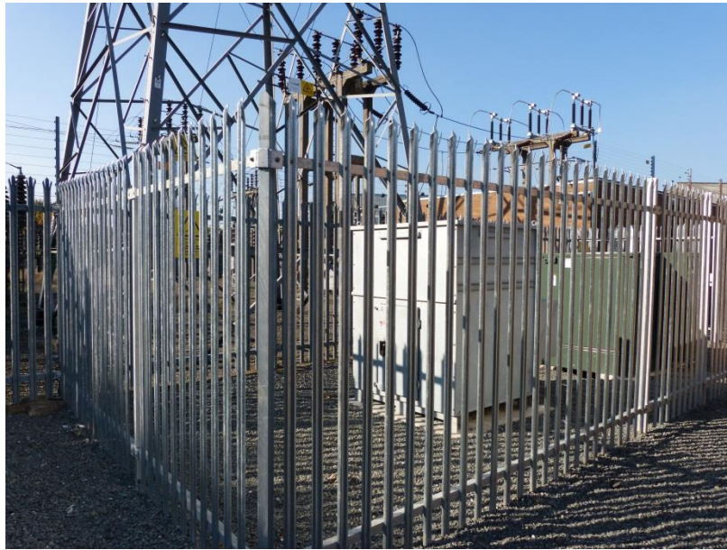
Figure 2-3 – Rear view of 11kV FLM
