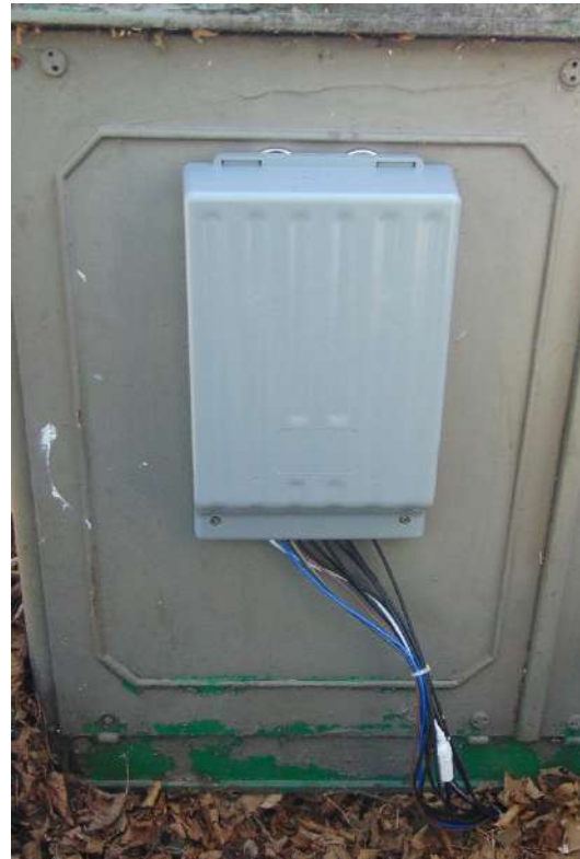
Figure 14: Lucy Electric GridKey MCU520 magnetically mounted in RR Wilmorton Substation
