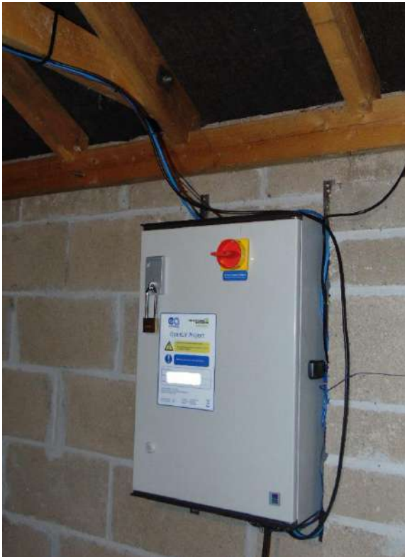
Figure 13: LV-CAP™ Enclosure wall mounted in Pilgrim Drive Substation
