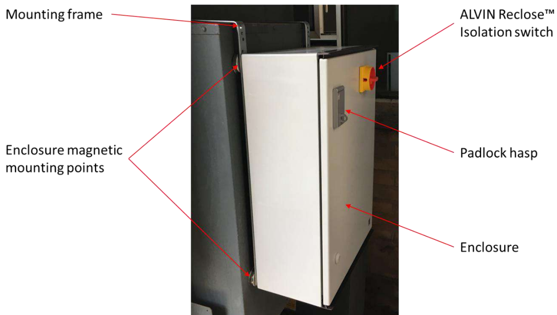
Figure 4: OpenLV Solution - Enclosure
