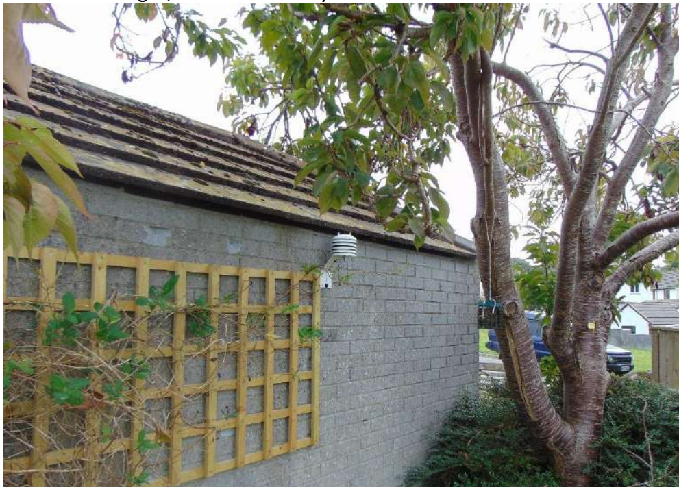
Figure 20: External Temperature Sensor and Radiation Shield at Pilgrim Drive substation
