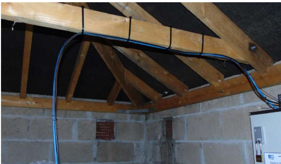
Figure 17: Cable routing in Chapel Street Substation
