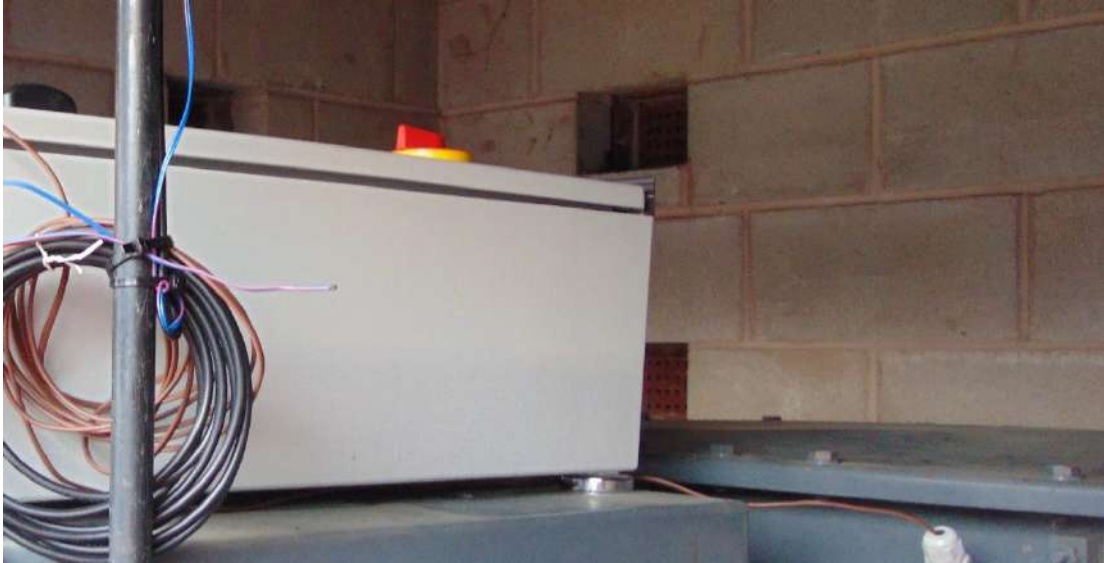
Figure 21: Internal ambient Temperature Sensor at Nuns Road Substation
