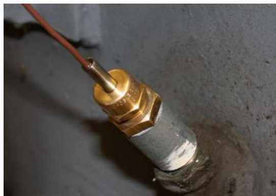
Figure 11: Example transformer oil pocket and test cap, including thermal probe
