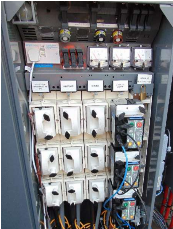
Figure 15: LV cabinet at Cosira Sleaford Substation
