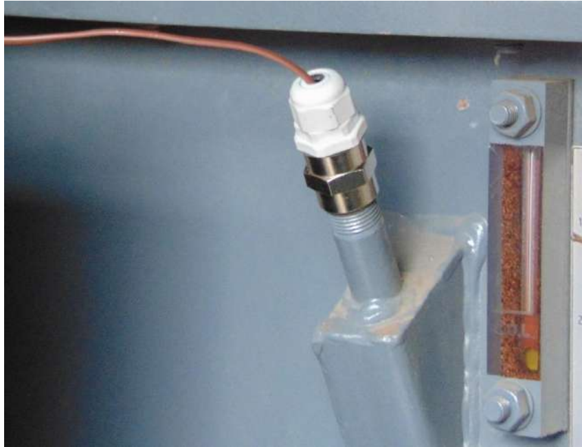
Figure 19: Thermocouple secured in Transformer Top-Oil pocket
