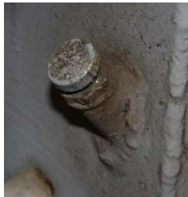
Figure 10: Example of a transformer oil pocket and cap
