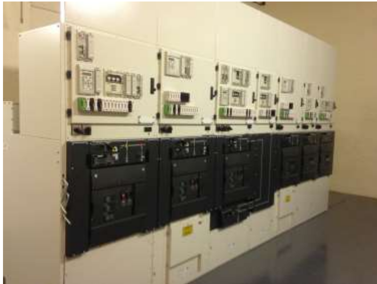
Figure 2-16 - New 5-panel Schneider switchboard
