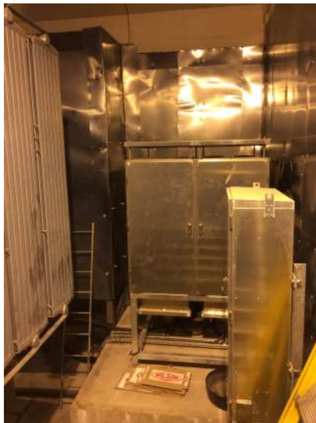
Figure 2-8 - FCL Control Cubicles and Shielding
