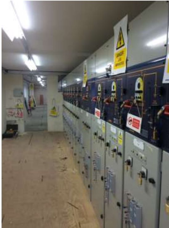
Figure 2-13 - Switchgear installed containing equipment for FlexDGrid
