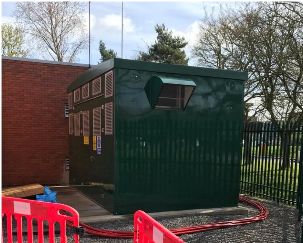
Figure 2-2 EDGE-FCLi installed in its final position at UoW
