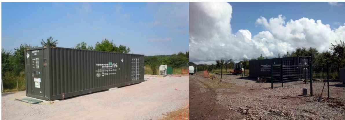
Figure 7: Battery on plinth before and after fencing
