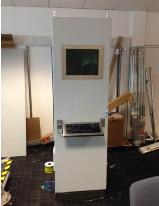
Figure 10: Local Control Panel
