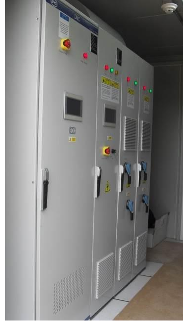
Figure 9: Circuit Breakers and Emergency Stop
