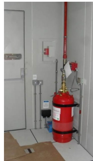
Figure 12: Fire Suppression Equipment
