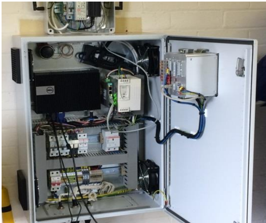
Figure 13: Power quality monitoring and communications equipment installed at Millfield Primary
