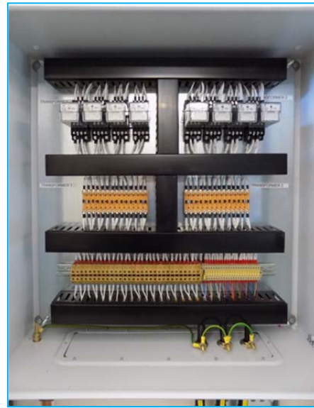
Figure 6-6 – MicroTAPP relay installation
