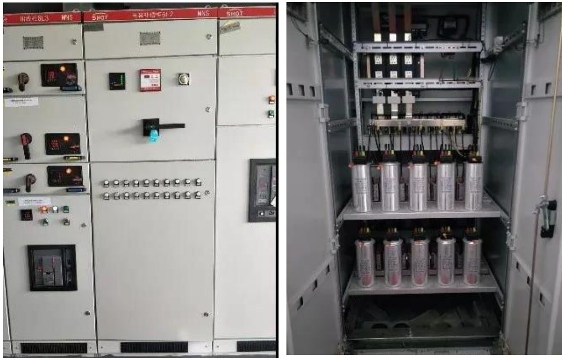
Figure 37: Front and rear view of AF designed by NANCAL, 3-phase, 400 V, 740 A [106].
