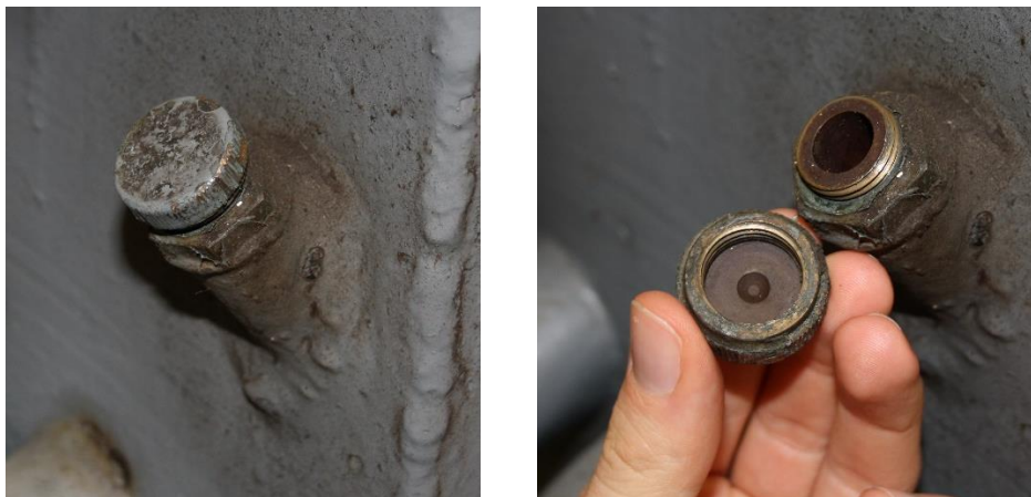
Figure 12: Example of a transformer oil pocket and cap.
