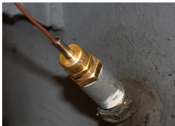
Figure 13: Example transformer oil pocket and test cap, including thermal probe.
