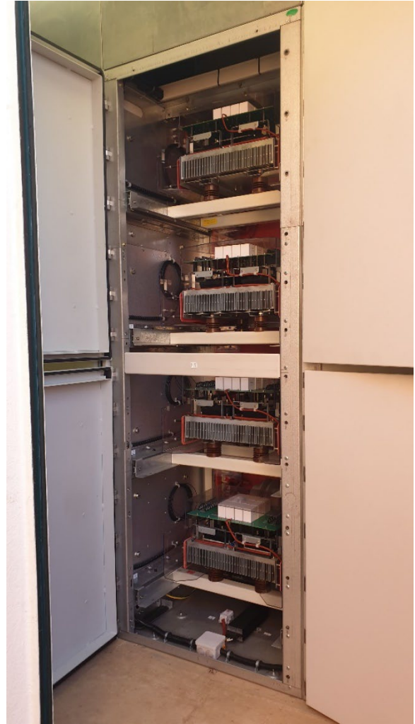
Figure 2-4 Image showing IGBT modules during visual inspection
