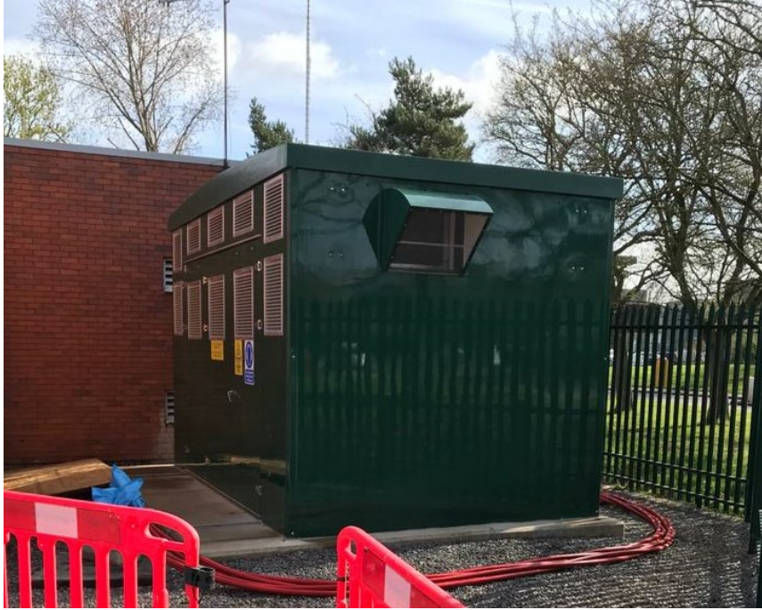
Figure 2-5 EDGE-FCLi GRP housing at UoW 33/11kV substation
