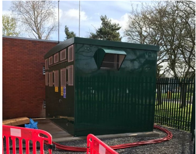
Figure 5-3 EDGE-FCLi in its GRP housing at UoW 33/11kV substation
