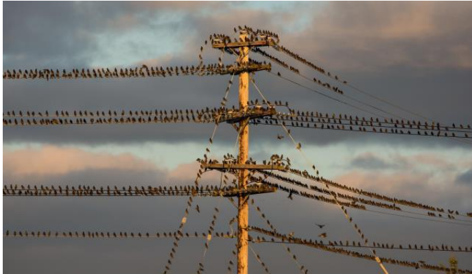
Figure 1 Electrical Interaction: Starlings on an 11kV section pole
