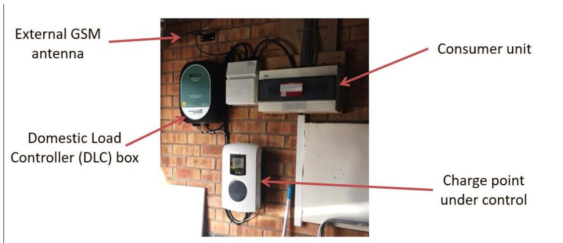
Figure 4.16 – Typical example of the EV charge point and DLC installation in customers’ homes
