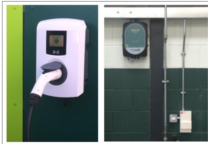
Figure 4.9 – Installation of controllable EV charge point and DLC representing customer-side equipment
