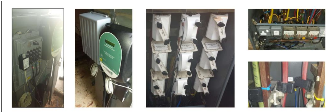
Figure 4.7 – Secondary substation equipment
