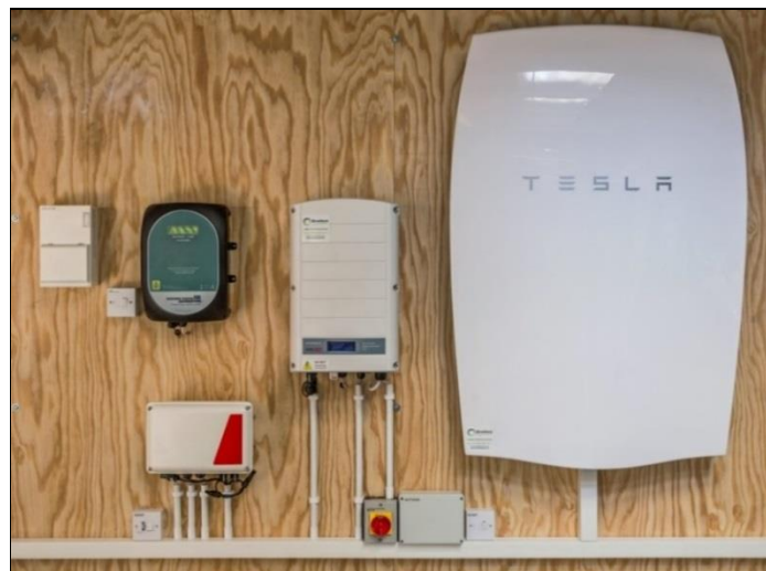
Figure 4.8 – Installation of battery, inverter and DLC representing customer-side equipment
