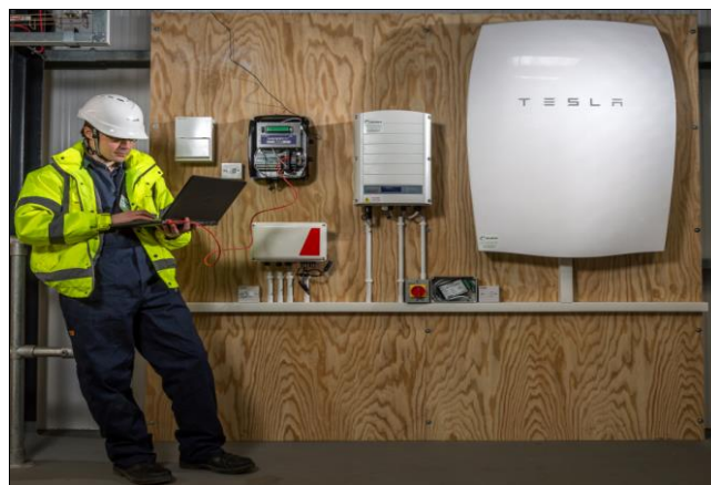
Figure 4.10 – Nortech engineer configuring the DLC box for export limitation tests
